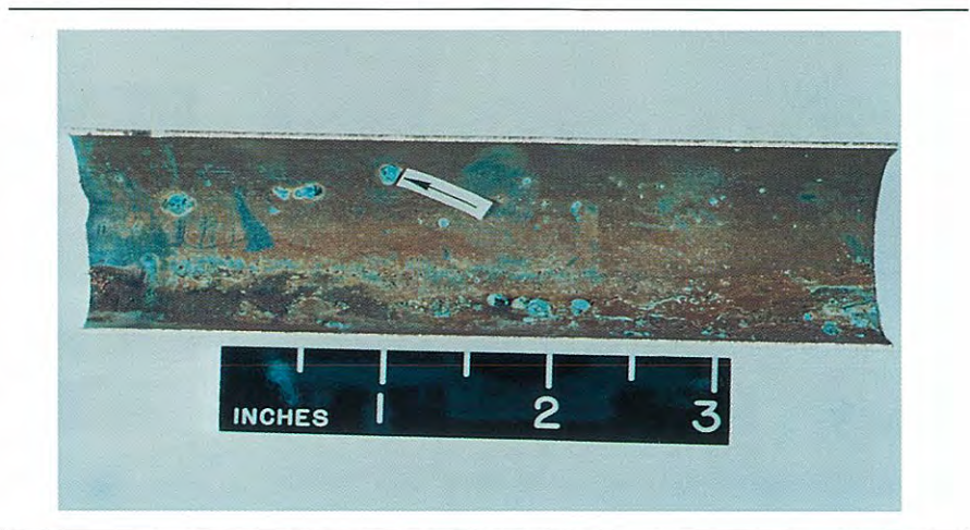
FIGURE 10 Hot water pitting corrosion of copper plumbing tube caused by the microdeposition of aluminum hydroxide (Al(OH) 3 ).
