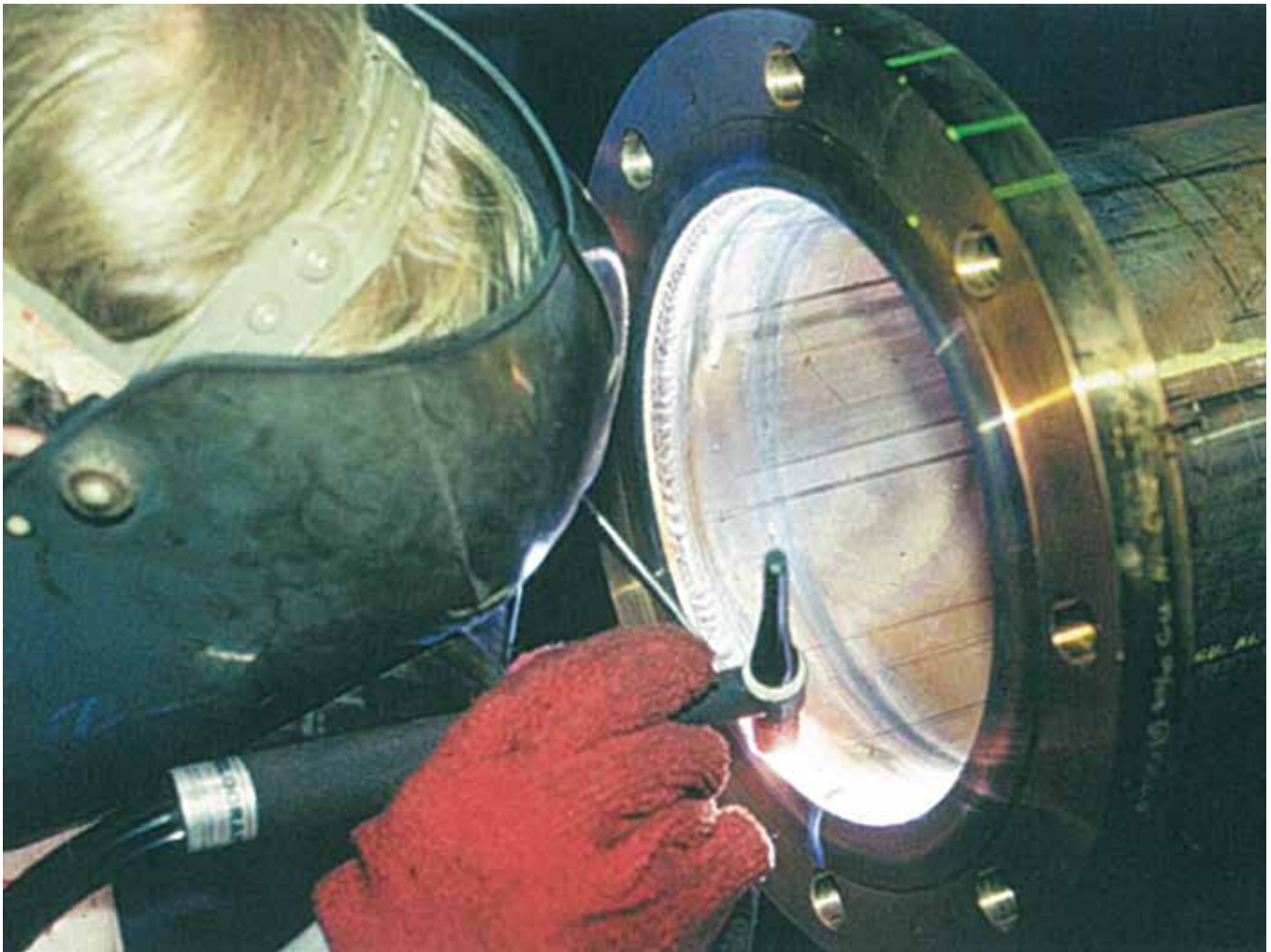
TIG welding 90-10 copper-nickel straight pipe to a bend (Courtesy of Eucaro Buntmetall GmbH)
