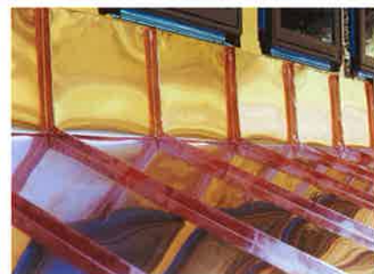
Some roofers use mechanical seamers, some hand seamers, and most a combination of the two. Copper forgives most scratches, and even oil canning is less apparent on dull, weathered copper. Below: Copper installers tend to use more precise details that other roofers never learned, like this pinch-seam transition detail on a home in Montana. PHOTOS, FROM TOP: PICKARD ROOFING; METALCRAFTS; MIKE WINTERS ROOFING
