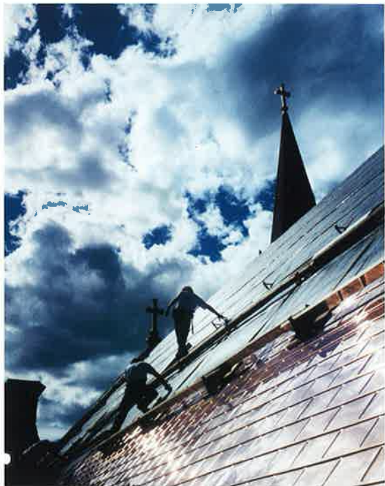
There's something special about copper projects. Re-roofing this 1901 church in Billings, Mont., with Revere's Bennington copper shingle got Bradford Roofing more comments than any other project. "It was a civic event," says Tom Bradford. BRADFORD ROOFING PHOTO
