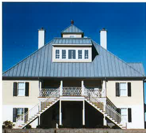
Lead-coated copper weathers to a flat pewter look that perfectly suits certain architectural styles and colors — like this North Carolina beach home. PICKARD PHOTO
