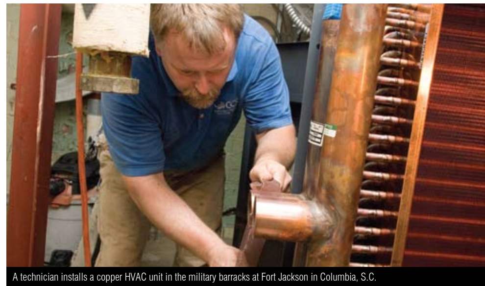
A technician installs a copper HVAC unit in the military barracks at Fort Jackson in Columbia, S.C.
