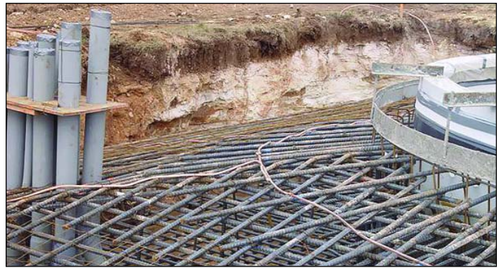
Figure 2. A ring of 250-kcmil copper is bonded to rebar in the footing skirt. The ring connects the conductors shown here with the ground ring shown in Figure 3 .
