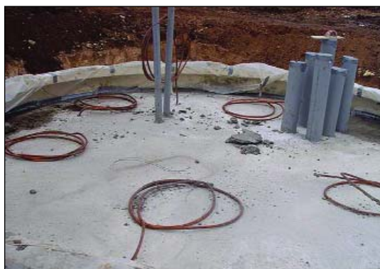
Figure 1. Central footing for a wind turbine tower under construction showing six 250-kcmil copper grounding conductors that will be bonded to the steel tower.
