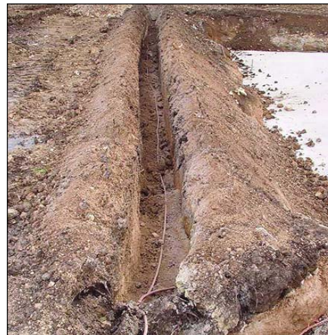
Figure 3. The footing skirt is encircled by a 250-kcmil copper ground ring, which, in turn, is bonded to four 8-ft copper-clad electrodes (foreground). Ground rings for all turbines are connected, again using 250-kcmil copper, thus establishing a uniform <1.5\text{-}\Omega ground potential for the entire wind farm.
