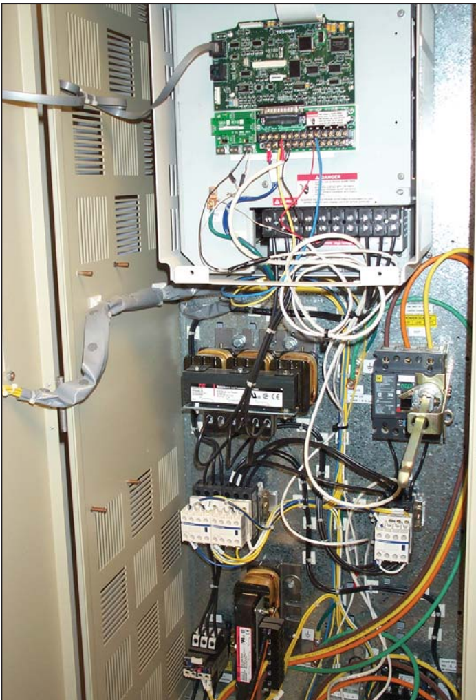
Figure 7. Variable frequency drives were installed on all blower and pump motors with variable torque loads larger than 7.5 hp. The VFDs addition to initial cost was easily made up by the energy they saved.
