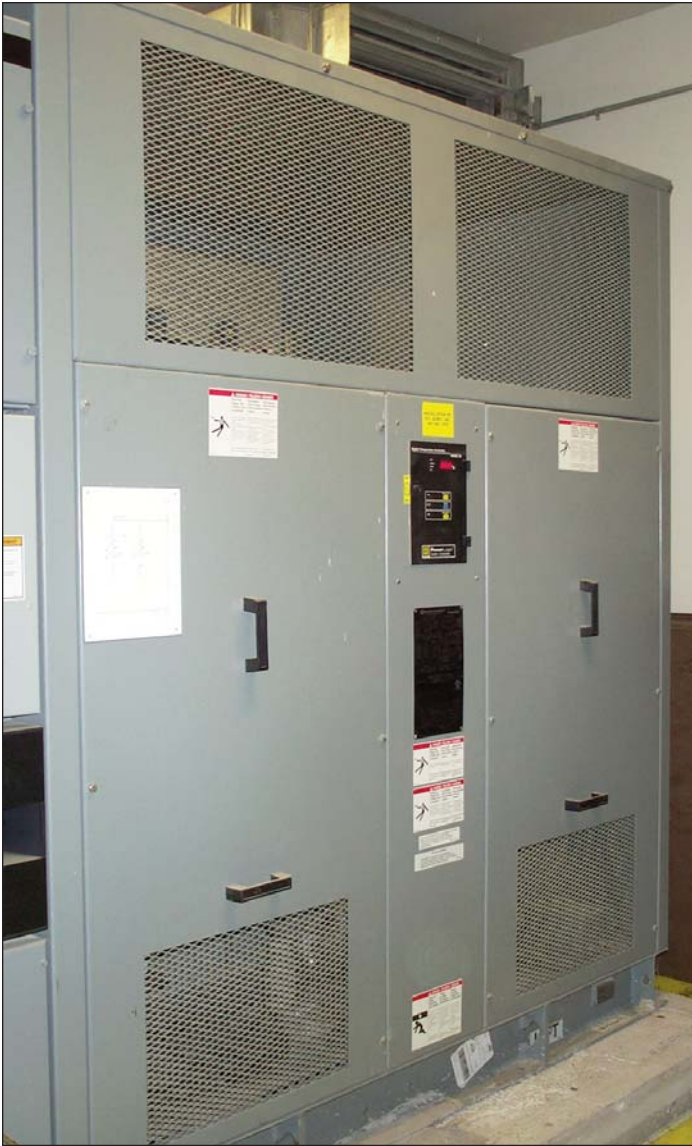
Figure 3. Two 750-kVA, dry-type, copper-wound transformers step down the local utility's unusual 12,470-V feed to 480/277Y service for distribution on campus. Copper was specified for efficiency and reliability.
