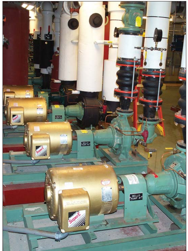
Figure 4. Four 25-hp Baldor Super-E premium-efficiency motors drive hot and chilled water pumps in the Bello Center. NEMA nominal efficiency of these motors is 94.1% at 100% power vs. only 89.8% efficiency for the 1970-vintage motors they replaced. Savings: $679 per motor per year; payback: 1.5 years.
