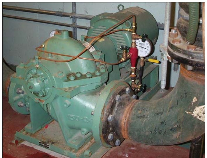
Figure 5. A 40-hp Baldor Super-E® motor drives a condenser pump in the Wellness Center. With a premium efficiency of 94.5%, the motor saved $1,069 per year over the standard-efficiency unit it replaced. Payback was only 1.5 years.
