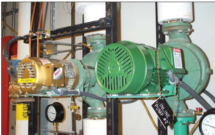
Figure 6. Two 2-hp premium-efficiency motors, operating continuously, replaced standard-efficiency motors and paid for themselves in 2.45 and 1.72 years, respectively.
