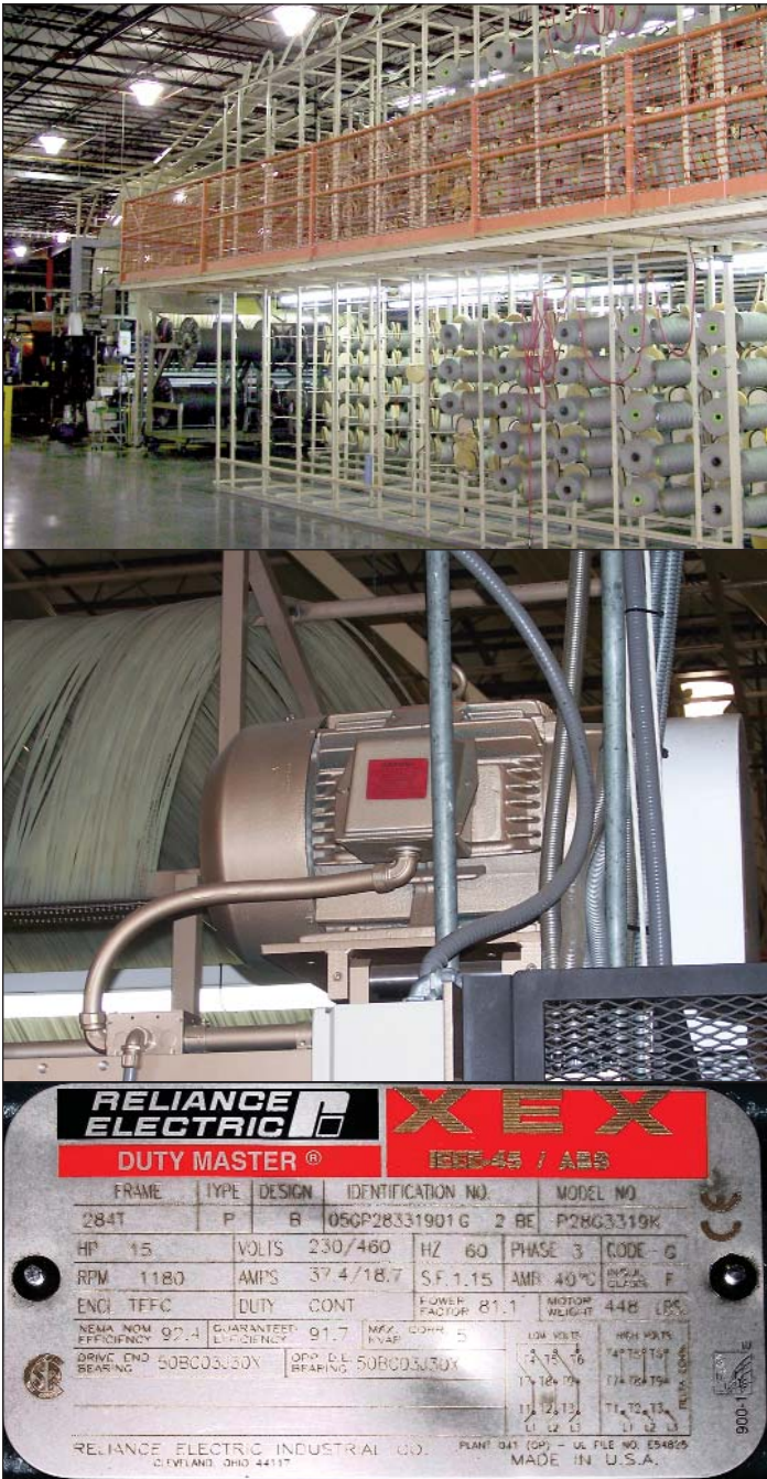
Figure 2. The pictures show a typical tufting machine (top), one of its two 15-hp, 1200-rpm drive motors (center) and a dataplate (bottom), which indicates that the motor's NEMA nominal efficiency is 92.4%. That level exceeds NEMA Premium standards, and the motor, therefore, satisfies Shaw's corporate policy.
