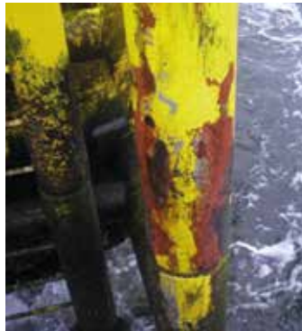
Several areas of damages on the boatlanding/steel surface.
