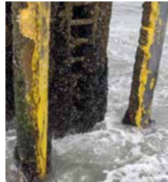
After several years the transition piece is completely covered with mussels and the ladder has disappeared amidst the growth.
