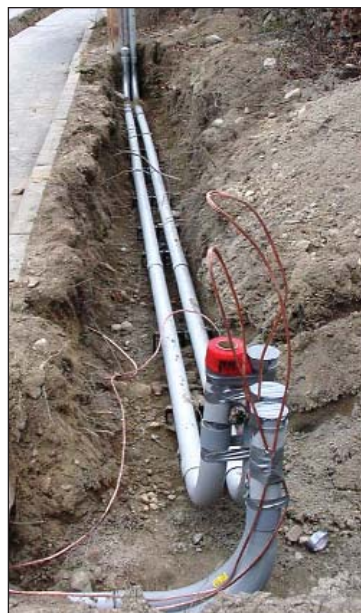
Figure 9. Because Bryant University is located on top of a small ridge and is subject to frequent lightning strikes, Bill Gilmore installed full copper ring-grounds around all high-voltage transformers. The additional copper ensures a robust, low-resistance ground for better lightning protection and exceeds code-minimum requirements.
