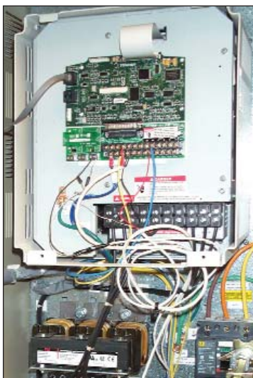
Figure 8. Harmonic-compensated reactors (lower left) trap harmonics generated by VFDs in motor circuits. The copper-wound reactors enable motors to operate cooler, quieter and at higher efficiency.
