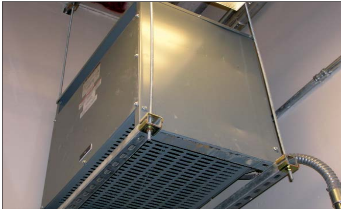
Figure 7. New K-rated transformers were suspended from overheads when the electrical system in Bryant's library was upgraded. The cool-running, all-copper transformers did not substantially add to heat loads in electrical closets.
