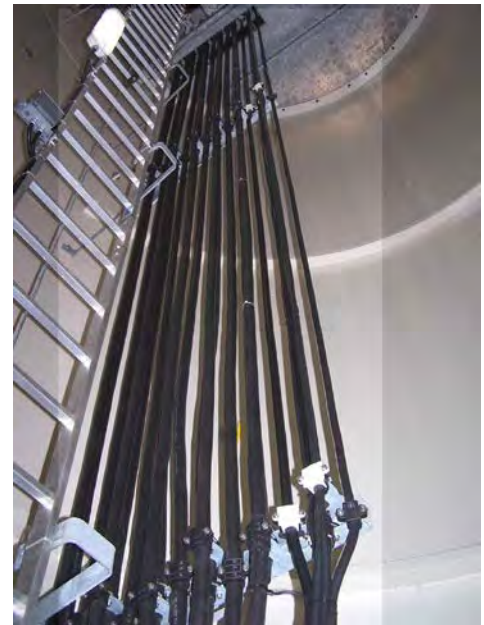
Figure 2. Heavy DLO cables inside the turbine mast transmit low-voltage generator power to switchgear and a step-up transformer.
