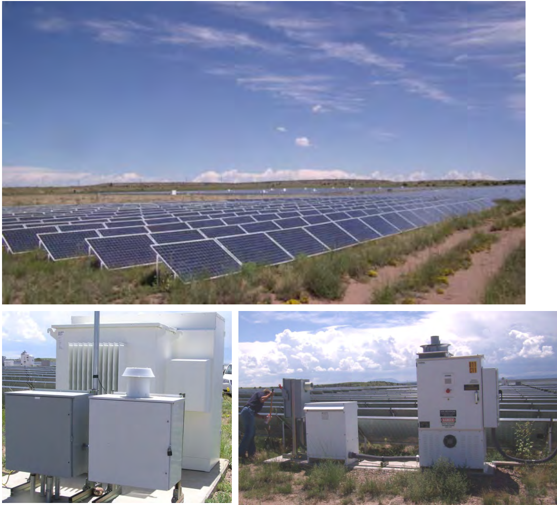
Figure 8. (Top) A portion of a 6.4-MW utility-scale solar field with panels arranged in rows. (Lower right) From right to left: One of the field’s 48 Inverters with attached dc disconnect connected to an intermediate step-up transformer and ac disconnect/meter. (Lower right) One of 12 large step-up transformers for transmission to the grid. Cabinets in foreground house instrumentation.
