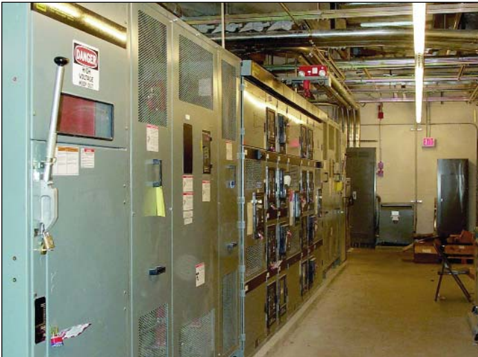
Figure 2. Transformers and controls in one of two double-ended substations serving the Stata Center. In each substation, a dual-rated (2000/2667- kVA), 13.8kV-480Y/277V, cast-coil, copper-wound, 115° C rise, Square D transformer feeds 480-V power to one of the towers via two copper buses. Lower floors have a more conventional architecture. Grounding connections from the main ground bus (not visible in photo) are made to a 500-kcmil copper ring ground that completely surrounds the building’s 1,400-ft perimeter.
