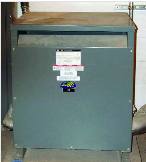
Figure 3. A 112.5-VA, 480V-208Y/120V distribution transformer, one of several installed on floors six through nine in the towers. Larger units are found on lower floors. The electrostatically shielded Square D transformers are copper-wound and contain low-loss silicon steel core laminations. They meet NEMA TP-1 efficiency standards and help reinforce MIT’s strong support for environmental stewardship.
