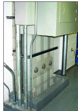
Figure 2. A 1,350-A/480-V copper bus duct leading from the Capitol Square basement to the building's utility loft on the 27th floor, from where it feeds the 300-kVA transformer that supplies 208Y/120-V service to the 17th through 27th floors. Aluminum feeder cables had loose connections, which contributed to the voltage drop experienced on the upper floors.
