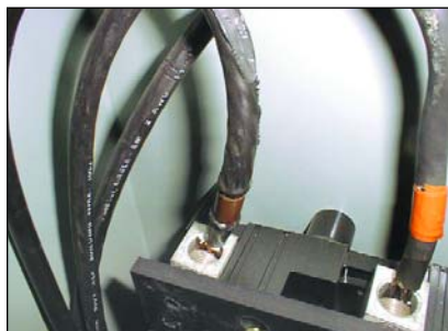
Figure 10. Evidence of overheating is seen in the damaged insulation on this aluminum conductor leading to the chiller disconnect switch on the building's 27th floor. The aluminum has been replaced with copper of the same wire gage.
