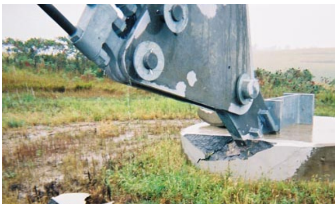
Figure 2. Damage to the outer "A" anchor from October 2003 strike. This event led to an upgrade of the entire facility's grounding and lightning protection system.
