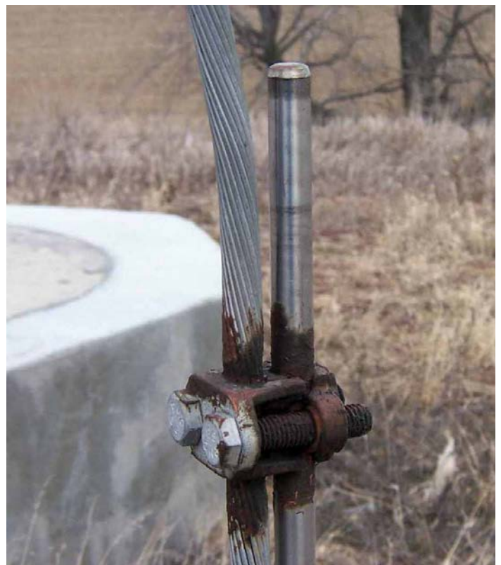
Figure 15. One of nine deep (up to 75 feet) grounding electrodes installed at the tower's guy cable anchors. The stainless steel electrodes were mechanically bonded to 250-kcmil tinned-copper conductors using approved, silicon-bronze mechanical connectors. The brown coating is a corrosion-resistant paint.
