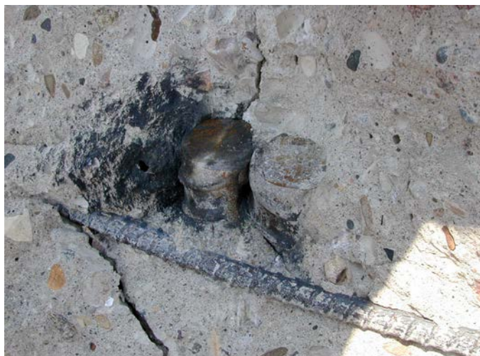
Figure 5. Burn scar on shattered concrete is evidence that lightning found a vertical reinforcing rod (center), which likely acted as an efficient Ufer ground, offering lower resistance than that of the installed grounding/lightning protection system.
