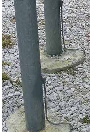
Figure 7. Two original AWG #2 copper grounding conductors were bonded to legs of the ice bridge. These and other existing grounds were retained and bonded to the new and more robust grounding system by CPC.
