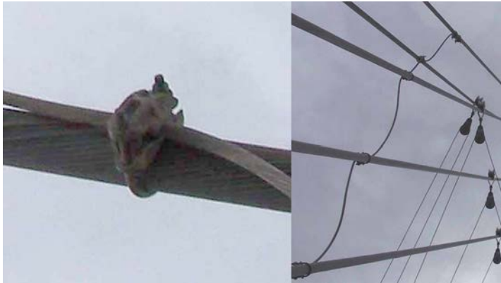
Figure 16. Approved, silicon-bronze connectors enable cables to run parallel at the point of contact, with orientation of the grounding conductors between guys at a narrow angle with the cables. (The pulleys seen at right are part of the cables' sway-damping system.)
