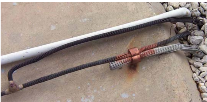
Figure 14. Existing and new grounding conductors at the tower were connected to create as large a system as possible. Here, new 250-kcmil tinned-copper grounding electrode conductors are crimp-bonded to old but still functional AWG #2 bare copper.
