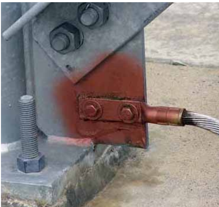
Figure 13. A 250-kcmil tinned-copper grounding conductor connected to an ice bridge leg. The ice bridge connects the tower and the KPTH transmitter building.
