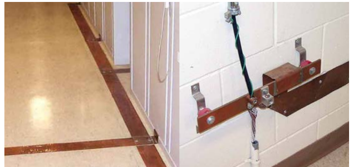
Figure 9. Grounding connections inside the transmitter building used flat-strip copper (left photo) connected via a ground bus (right photo) to the outdoor electrode field.
