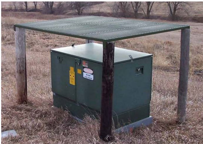
Figure 17. The site's 13-kV utility switch was protected with its own deep grounding electrode, marked by the orange conduit at lower left in the photo. This electrode interrupts and shunts to ground any surges resulting from lightning strikes on the nearby power grid.
