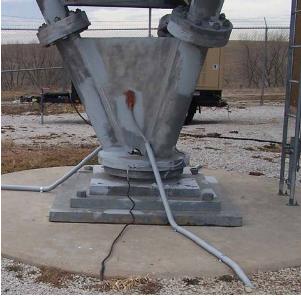
Figure 6. One of two original AWG #2 copper ground leads at the tower base (foreground, bare wire) were augmented by three new 250-kcmil tinned copper conductors (two shown, in protective sleeves).
