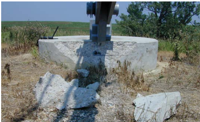
Figure 1. Lightning damage to the outer "B" cable anchor from a June 2001 strike. The strike ejected 100-lb blocks of concrete several yards from the anchor after bypassing the existing high-resistance grounding system.
