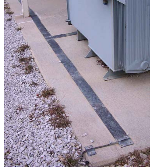
Figure 8. Existing flat-strip copper grounding conductors, used with transformers and other outdoor equipment, were retained and bonded to the new system (large conductor in foreground). The existing outdoor grounding system was also tied into these strips (not shown).
