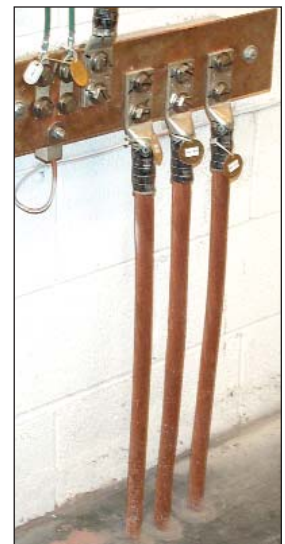
Figure 7. Penetrations through floors are lined with PVC to avoid the risk of fire. Metallic penetrations can suffer hazardous resistive heating when large surge currents pass through the grounding conductors. Connection lugs are tinned copper.
