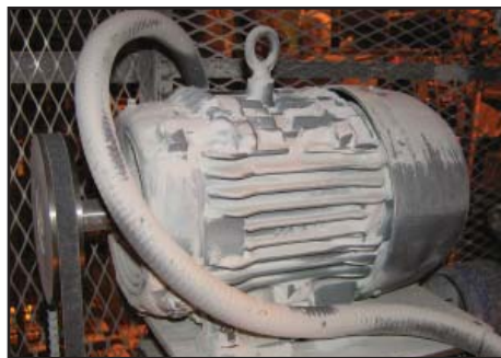
Figure 2. A mineral-dust-covered blower motor at Willsboro illustrates the plant's need for IEEE 841 Severe Duty motors. IEEE 841 motors also meet NEMA Premium efficiency requirements, but Siemens copper-rotor Ultra Efficient Motors exceed those standards.
