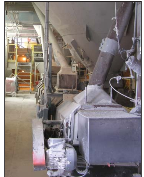
Figure 3. A 2-hp SE&A IEEE Plus belt conveyor motor (lower right of photo) that transports finely-ground product to the beneficiation department. It was one of the first copper-rotor motors installed during the current replacement program. The data plate lists the motor's NEMA nominal efficiency at 87.5%, one full percentage point higher than called for under NEMA Premium standards.
