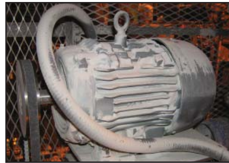
Figure 2. A mineral-dust-covered blower motor at Willsboro illustrates the plant's need for IEEE 841 Severe Duty motors. IEEE 841 motors also meet NEMA Premium efficiency requirements, but Siemens copper-rotor Ultra Efficient Motors exceed those standards.
