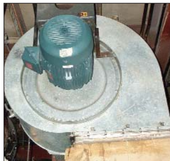
Figure 1. A 20-hp NEMA Premium motor drives a blower at Kodak Park. According to MotorMaster+, the motor saves the company 4,200 kWh and $315 per year compared with rewinding the standard-efficiency motor it replaced. This one small motor reduces annual carbon dioxide emissions by more than 5,400 pounds per year. Payback time for the new motor was only 1.1 years.
